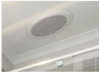
9 Ceiling exhaust fans above showers and to any wet areas without external ventilation
